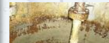
Dirty tanks with hardened products before cleaning.
