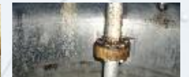
Cleaned tanks after full automatic cleaning procedure.
