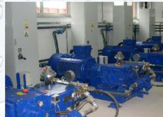
Machine room tank interior cleaning of rail coaches 800 bar.
