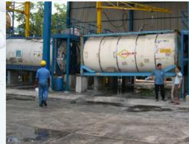
Tank cleaning station for interior cleaning of tank containers.
