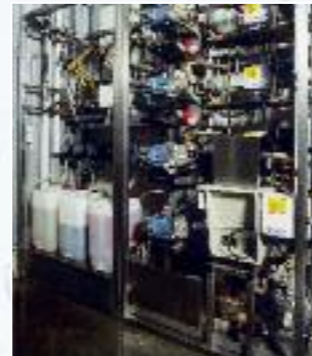
4 pump equipment with different dosing system.
